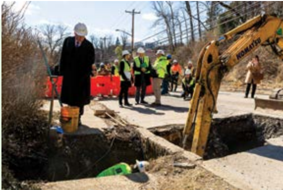
Principal Deputy Assistant Administrator for the EPA's Office of Water Bruno Pigott watches as crews replace a lead service line on Hazelwood Avenue.
