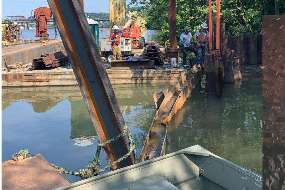
Setting up to build the steel sheet pile cofferdam on the Monongahela River
