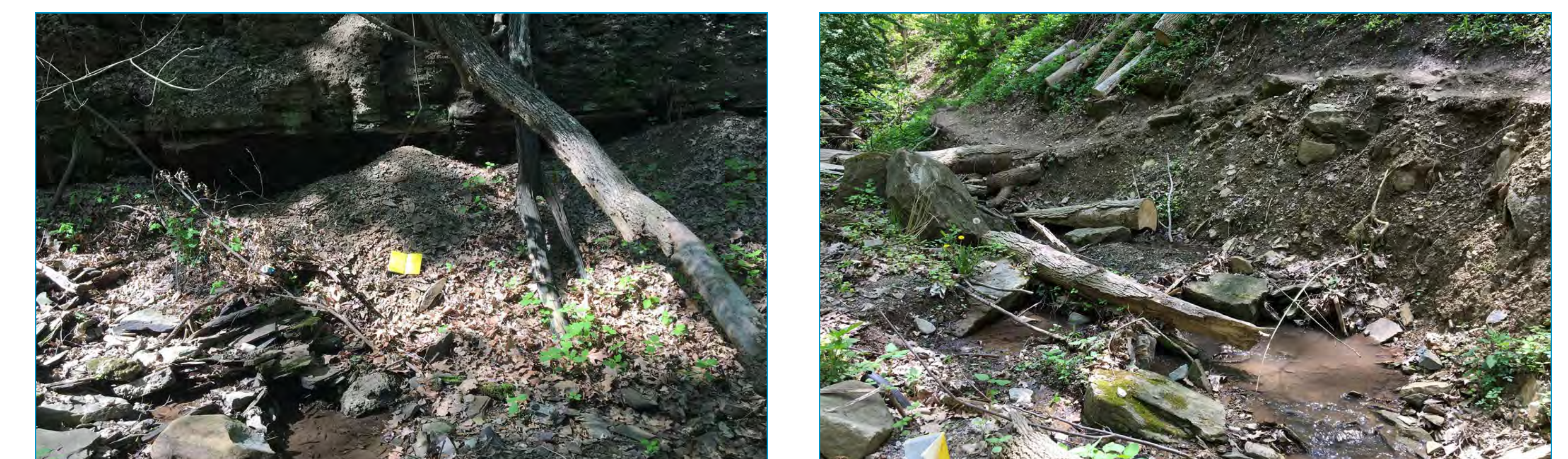
Erosion can wash out trails and fill streams with gravel and debris.
